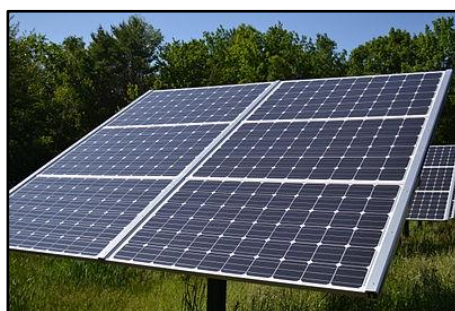
Plaques solar fotovoltaiques. 15
